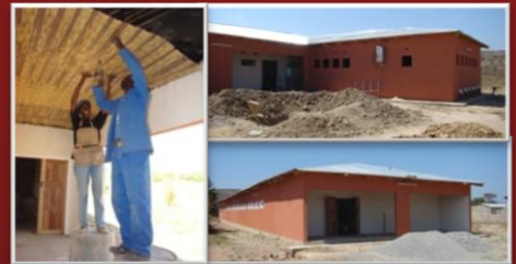
Installation of ceiling and external painting complete on the orphanage building for New Beginnings, Kafue
